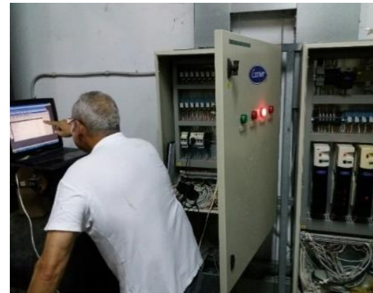
Carrier - HVAC BMS automation configuration
